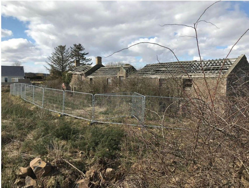
Figure 3: Quarry buildings at Embleton quarry, now in a state of disrepair
